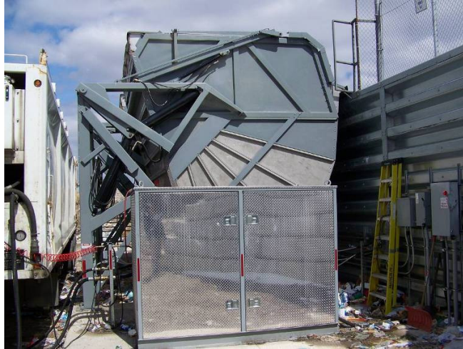
Photo 9 – Side view of Transtor Units (Note bin wall configuration and electrical/hydraulic installations)
