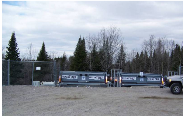
Photo 6 – Two Transtor Units at Dryden Transfer Station
