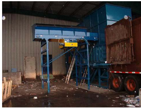
Photo 10 - Hopper and Conveyor for Containers
